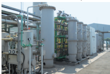
PSA process bench plant
