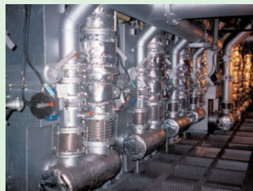
Reheating furnace with regenerative burners
