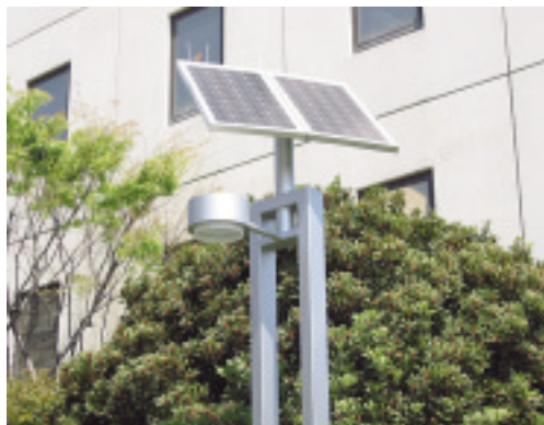
Solar street lights installed at the Tsurumi Engineering and Manufacturing Center
