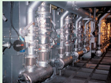
Reheating furnace with regenerative burners
