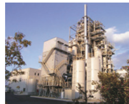
Biomass boiler system
