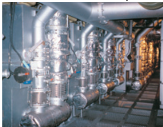
Installation status of regenerative burners
