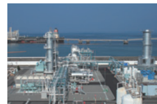
VOC recovery equipment
