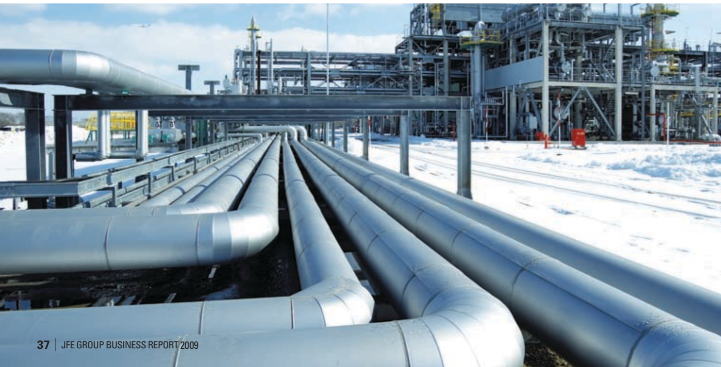
Natural gas plant
