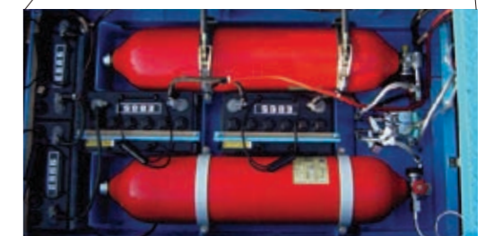
Hydrogen gas tanks up close (under the cargo bed)
