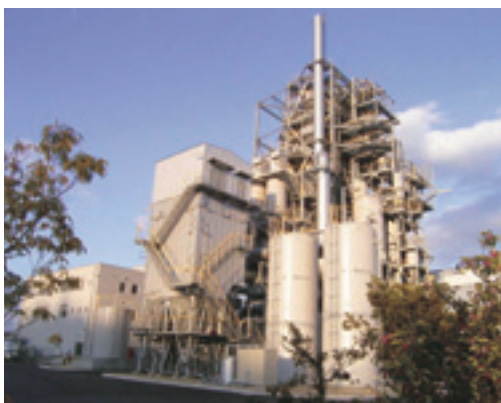
Biomass boiler system
