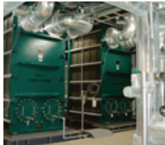
Air-Conditioning System Using Clathrate Hydrate Slurry
