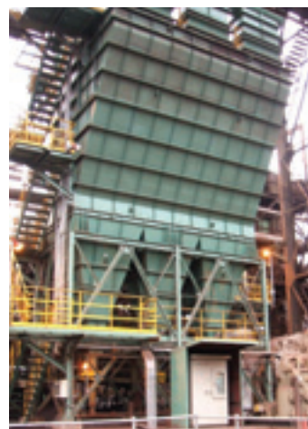
Dust collector at West Japan Works (Fukuyama)
