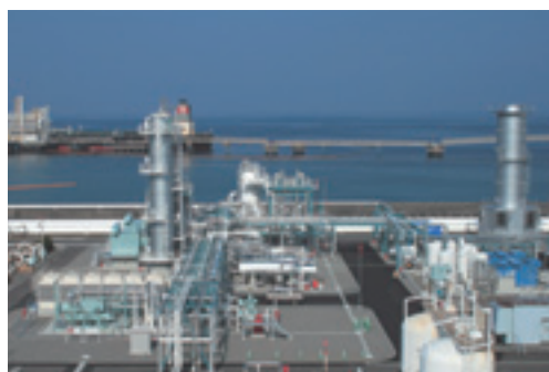
VOC recovery equipment
