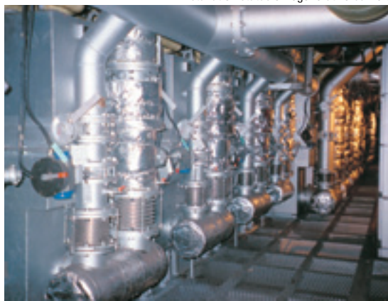
Installation status of regenerative burners
