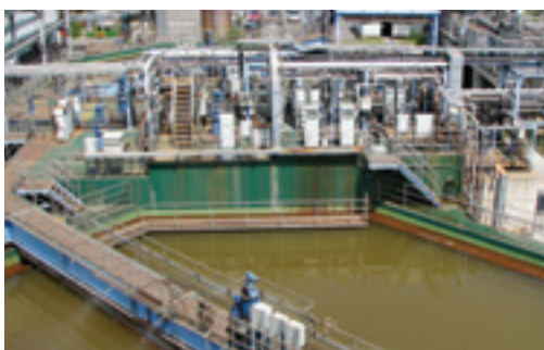
Water treatment facility at East Japan Works (Chiba)
