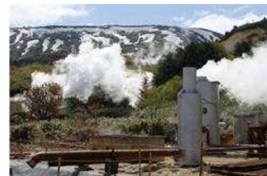
Geothermal Power Station
