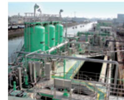
Wastewater treatment: Denitrification equipment at East Japan Works (Chiba Area)
