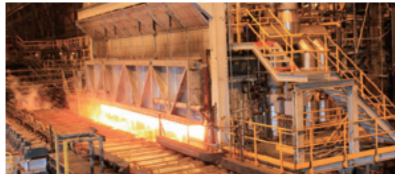
CSI's No. 5 reheat furnace
