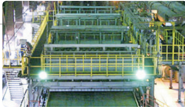
Super-SINTER® system Keihin District plant
