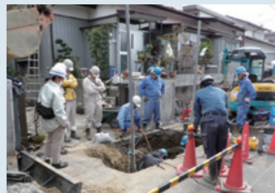
Check and repair of gas pipe channels in Sendai immediately after the earthquake
