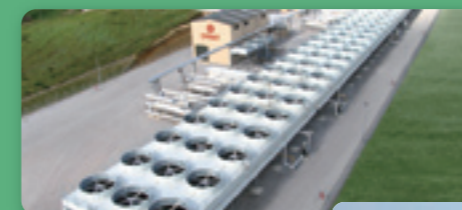
Geothermal binary power generation based on low-temperature steam and hot water (JFE Engineering, page 43)
