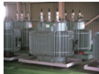
Warehouse of PCB equipment and its equipment storage status West Japan Works (Fukuyama Area)
