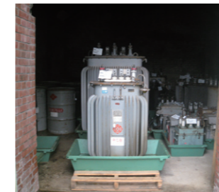
Storage of PCB transformers at Maizuru Shipyard
