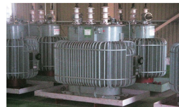
PCB storage equipment in West Japan Works (Fukuyama District)
