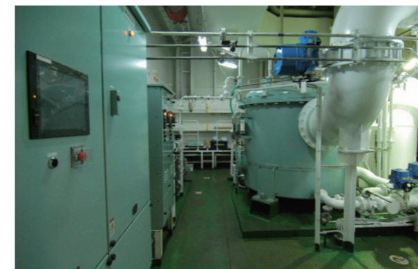
JFE Ballast Ace (filter and control panel)
