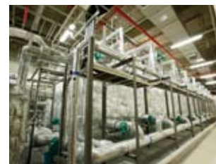
Neo White® Clathrate hydrate slurry (CHS) heat-storage air conditioning system at Tsurumi Works
