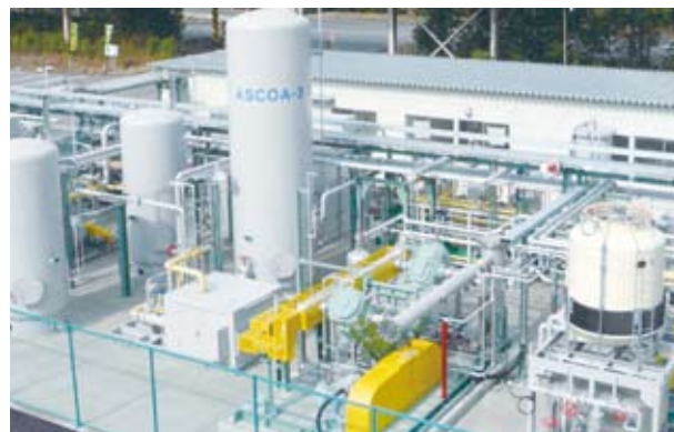
Experimental equipment for separating CO 2 using PSA (Fukuyama District)
