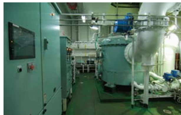
JFE Ballast Ace (filter and control panel)
