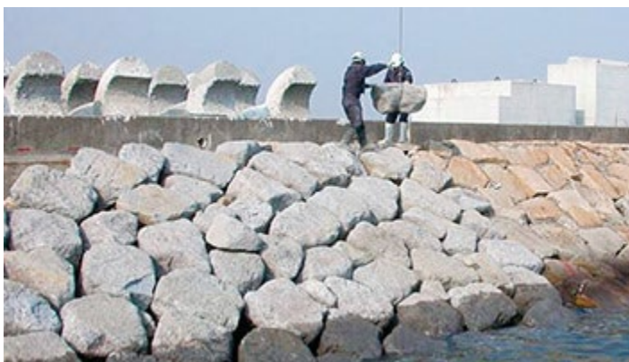
Coastal construction work using artificial stones made from steel slag hydrated matrix
