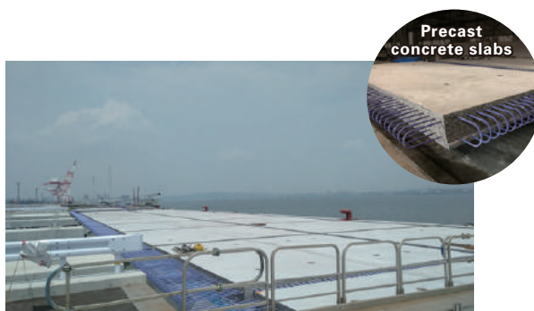
Precast concrete slabs mixed with finely ground blast furnace slag installed in piers
