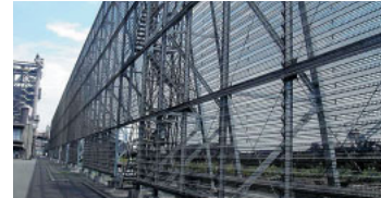
Windbreak fence in West Japan Works (Kurashiki)
