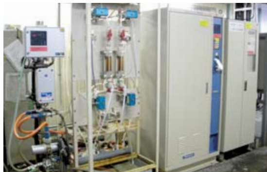
Automatic wastewater analyzer: an example from East Japan Works (Chiba)
