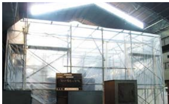
Oil removal test for large devices
