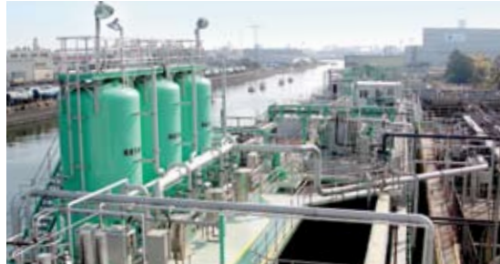
Wastewater treatment equipment: Example of denitrification equipment for wastewater at the East Japan Works (Chiba)
