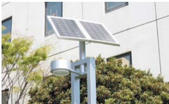
Solar street lights
