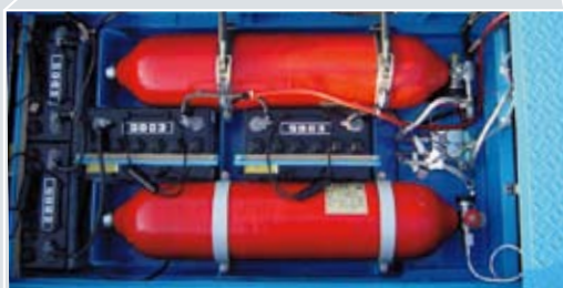
Hydrogen gas tanks up close (under the cargo bed)
