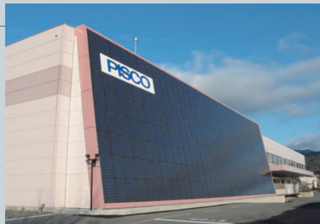
Example of a solar panel installation (Ina No. 2 Plant of Nihon PISCO Co. Ltd.)
