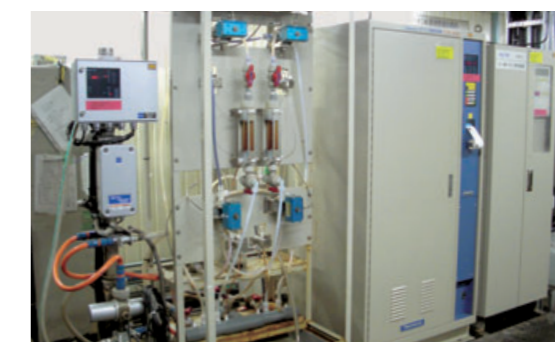
Automatic wastewater analyzer: an example from East Japan Works (Chiba)
