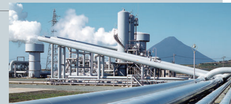
Yamakawa Geothermal Power Station (Ibusuki City, Kagoshima)
