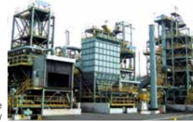
Ferro-coke production facility
