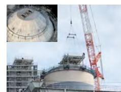
Example of reducing work in high locations by using high-precision 3D measurement data generated with drones
