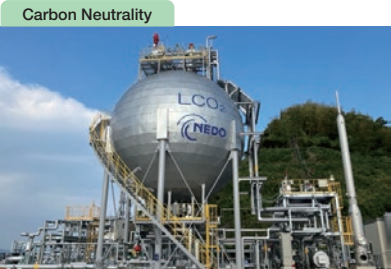
CO 2 transportation system (onshore facility) at The Kansai Electric Power Co., Inc.'s Maizuru Power Station We provide integrated services from design through construction of world-leading facilities.
