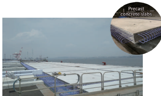
Precast concrete slabs mixed with finely ground blast furnace slag installed in piers
