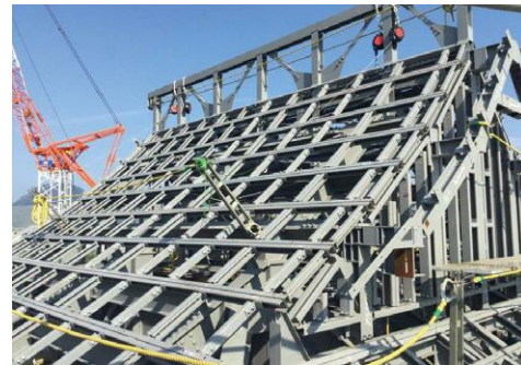
Steel construction of the six-story of the castle tower of Kumamoto Castle
